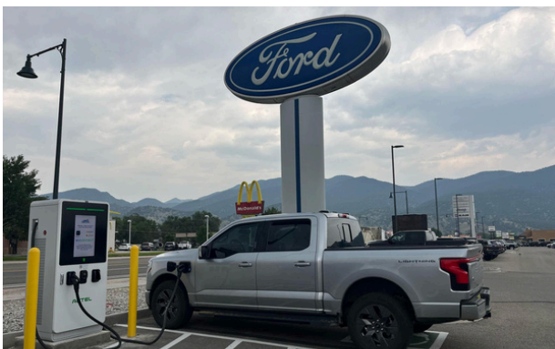
Source: PlugShare, EV charging station at Salida Faricy Boys
